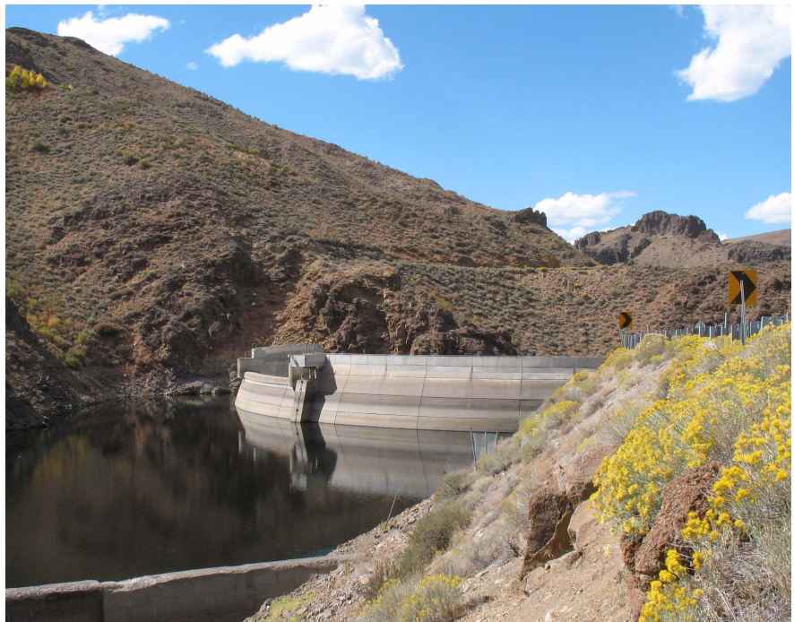
Photo 5.10. Wild Horse Reservoir is impounded behind a double-curvature arch dam completed in 1969 to replace the original dam, Nevada
